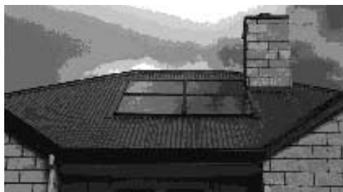
Insitu Pumped Flat Plate System collector
