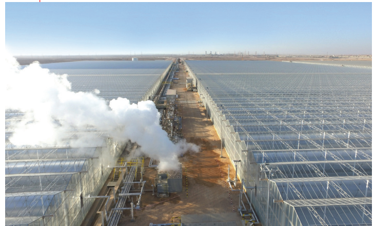
▲ The world's largest solar process heat plant Miraah in Oman was significantly enlarged in 2019 and now has an installed capacity of 300 MWth. Photo: GlassPoint Solar, Inc.
