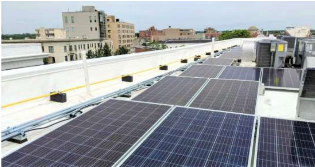
Figure 5: Solar arrays at the Maycroft Apartments complex. Credit: New Partners Community Solar, 2022.
